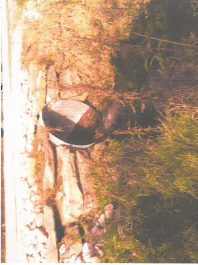
Round the Pond Rd. (at Greenwood Rd. intersection) 72" CMP - POOR
