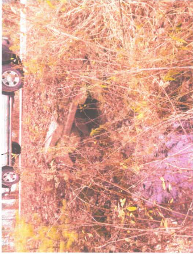
Pleasant St. (between Maple St. & Hayden Ave.) 42" CMP - POOR
