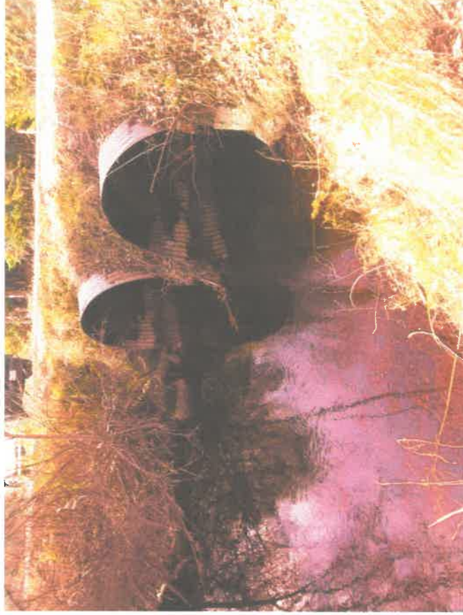
Emerson Rd. Twin 72" CMP - FAIR (starting to rust)
