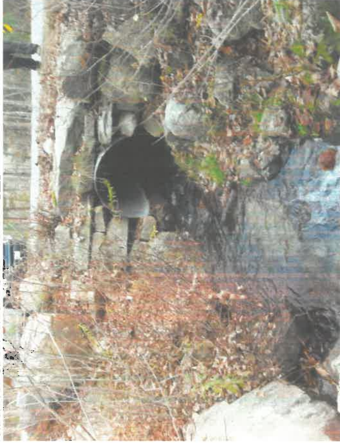
Sodom Rd. (Sand Pond (outlet brook) 60" CMP - POOR
