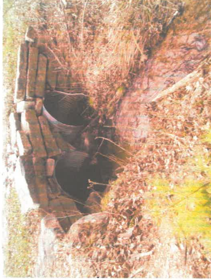
Shedd Rd. Twin 48" CMP - GOOD (installed 2012)
