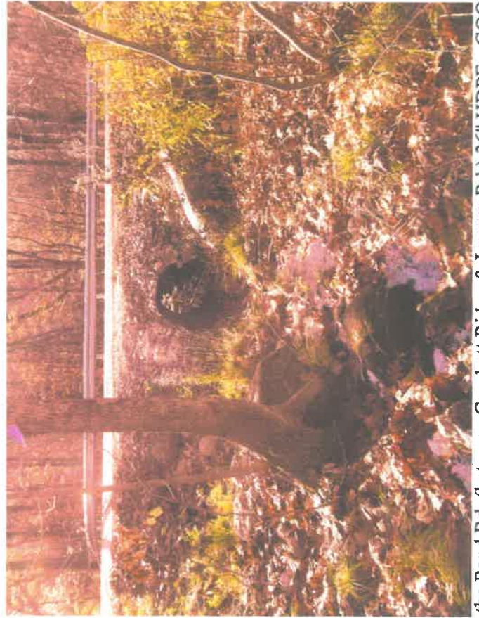
the Pond Rd. (between Crockett Ridge & Larson Rd.) 36" HDPE - GOOD
