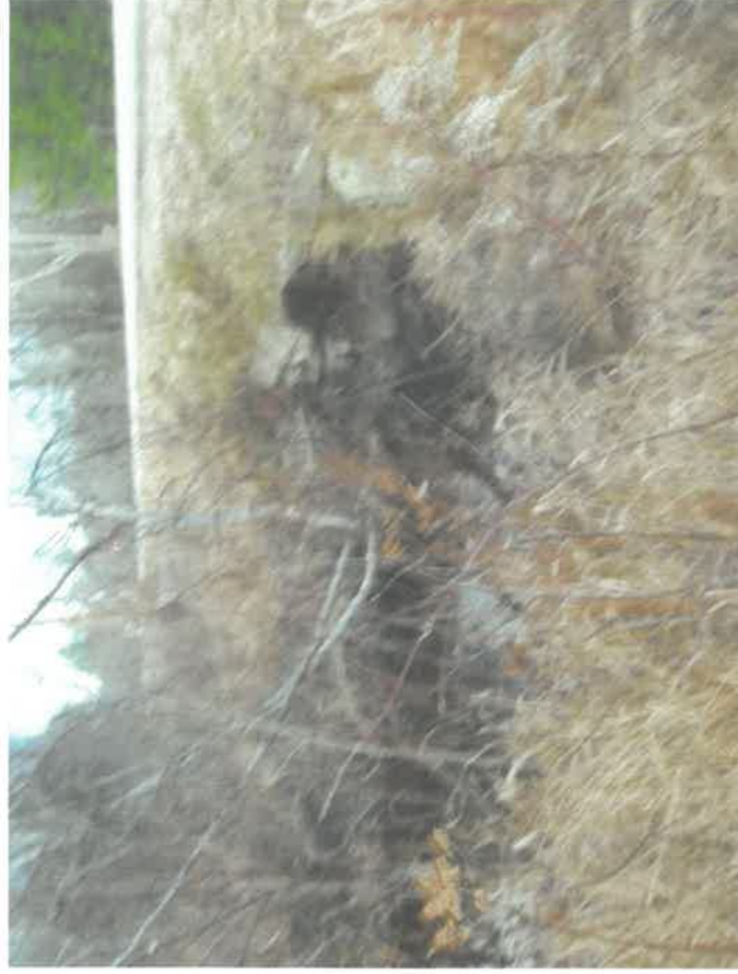
(Photo 1 of 2) Town Farm Rd. twin culverts (above 7' boiler steel plate) - GOOD
