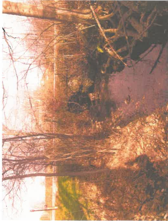
Greenwood Rd. (at Morse Rd.) 48" HDPE - GOOD
