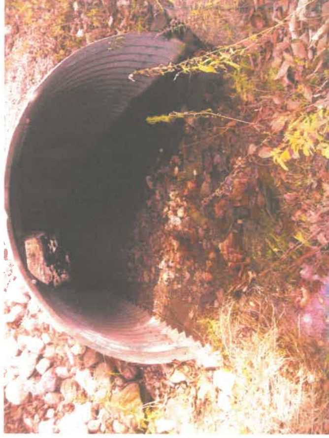
Greenwood Rd. (old State section) 100" multi-plate extended to concrete box - GOOD Page 2 of 6
