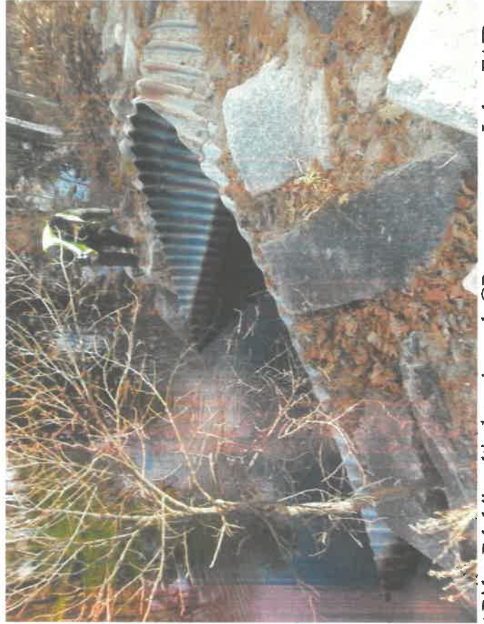
Ridge Rd. 14' multi-plate pipe arch @Pennesseewassee Lake - FAIR
